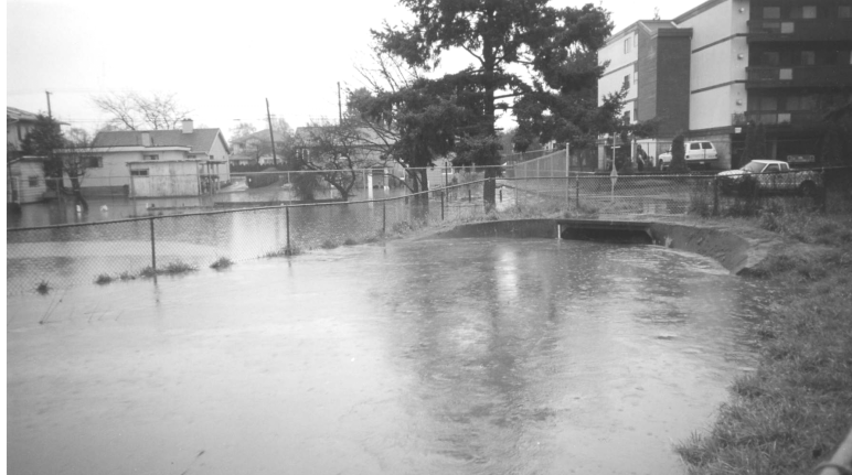
Figure 6. Looking downstream from the Bowker Creek culvert under the intersection of Fort Street and Foul Bay Road during a flood. Note the affected nearby residential properties. December 1999.
